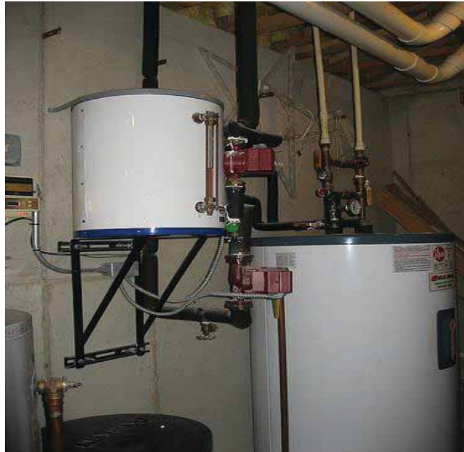
Figure 13(a): A solar hot water system accessed from Flickr, 2011.
